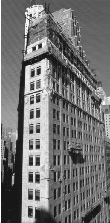
PHOTO: Over 100,000 lbs. of PUMP-X53 were pumped into wall cavities between terra cotta and rubble masonry back-up on this building on Wall Street in New York City as part of a masonry stabilization project.
