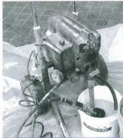
PHOTO: Airless sprayer, adapted for pumping of PUMP-X53i . Spray gun was removed and replaced with a ball valve and adaptor, bushed down to 1/8 " diameter tubing. A rubber seal, set 2-3" above end of tubing, prevents grout from running out of injection port.
