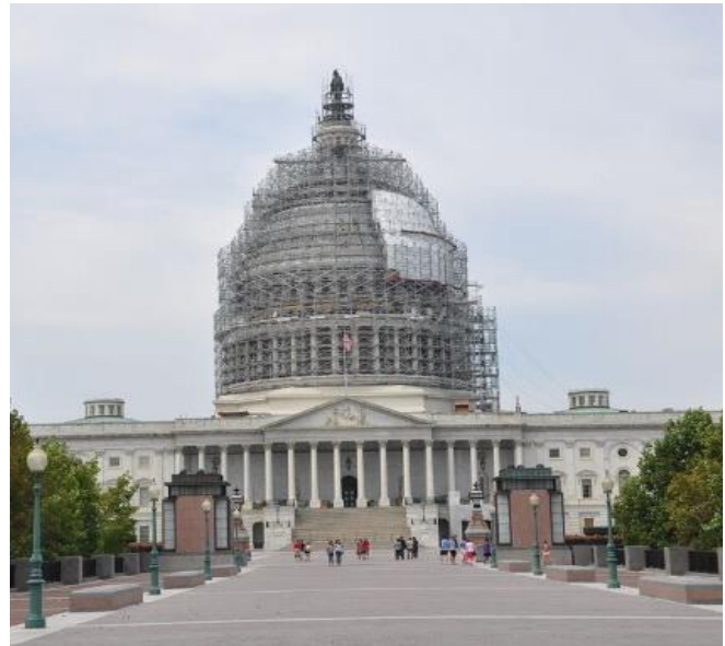
Photo: Edison Coatings LP-20 lime putty was used in the repointing of the masonry base of the U.S. Capitol Dome.
