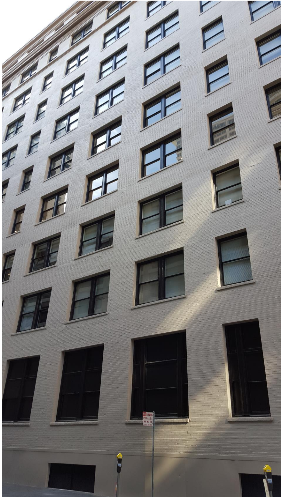
Rear elevation, one year after consolidation with System 95W and coating with custom-matched Elastowall 351.
