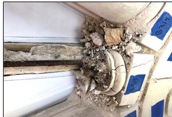
Spoke removed to reveal steel corrosion
