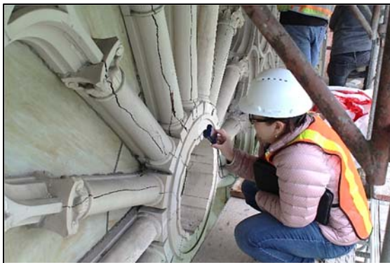
Inspection of cracked Rose Window tracery
