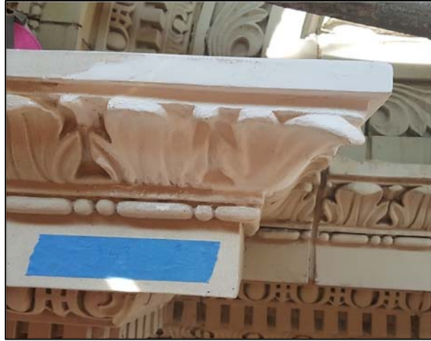
Porch cornice return recreated, part-way through restoration, awaiting additional carving and coatings
