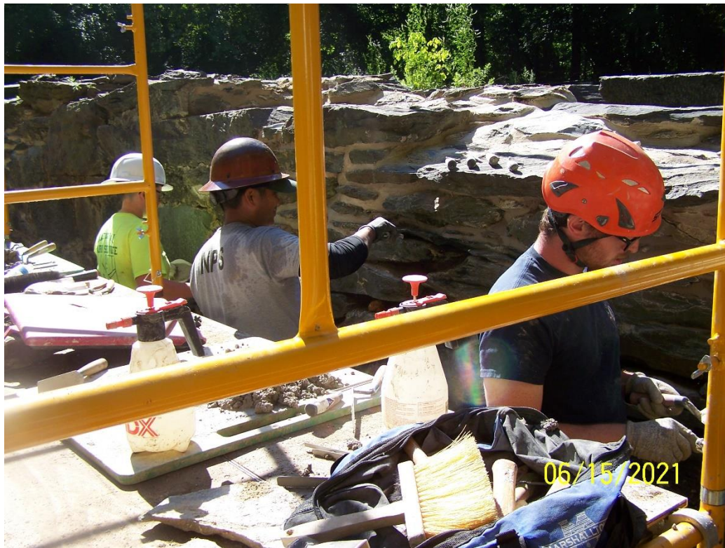
HPTC Masons install Rosendale 12M natural cement mortar at the Pulp Mill Ruins.
