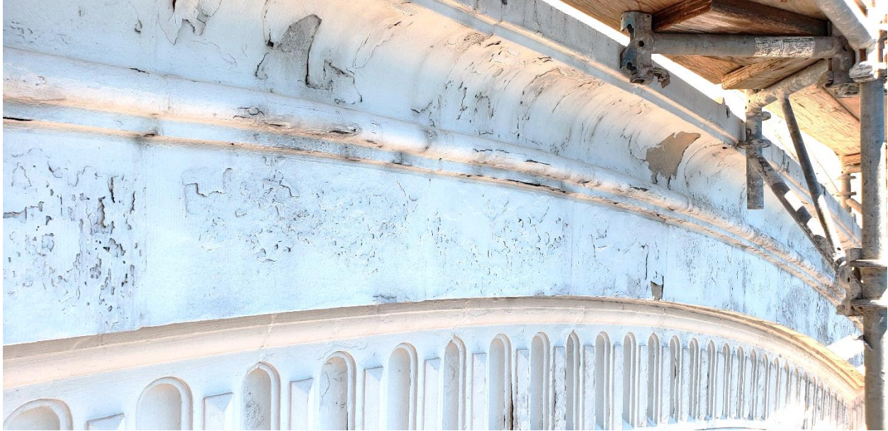
Figure 5. Widespread glaze spalling, just below the roof level, north facade, 2018
