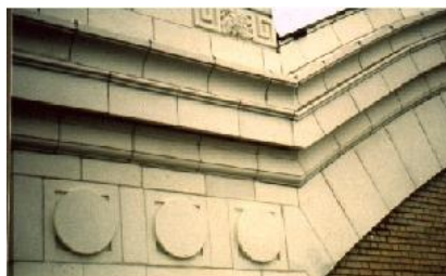
Figure 2. Section at the top of the North elevation, before and after repair in 1998.
