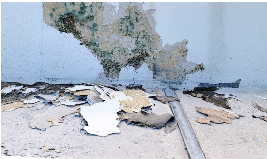
Figure 6. Glaze spalls reveal biological growth in wet masonry on north elevation parapet.
