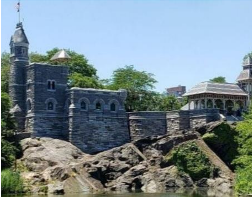
Belvedere Castle, New York City Central Park: Skyward facing mortar joints on coping stones were restored using BioMix 50 and ICE MINUS 9 (RL-9) from 2018-2019.
