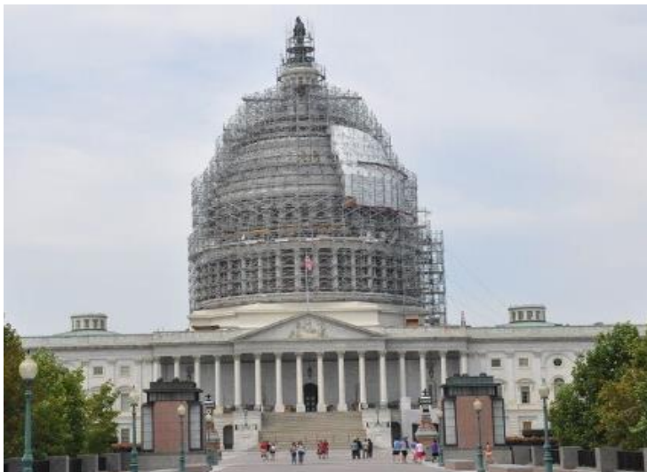
Photo: US Capitol Building, Washington, DC. Multiple colors of Rosendale 13P Type L were used for patching the exterior marble.
